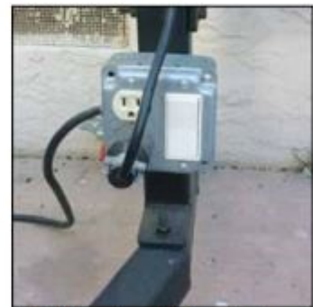
4 Switched outlet for safety. □
